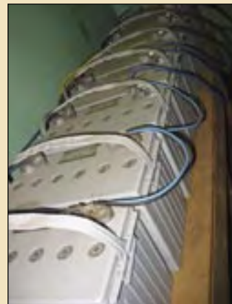
Battery banks provide additional power during surges and outages.
